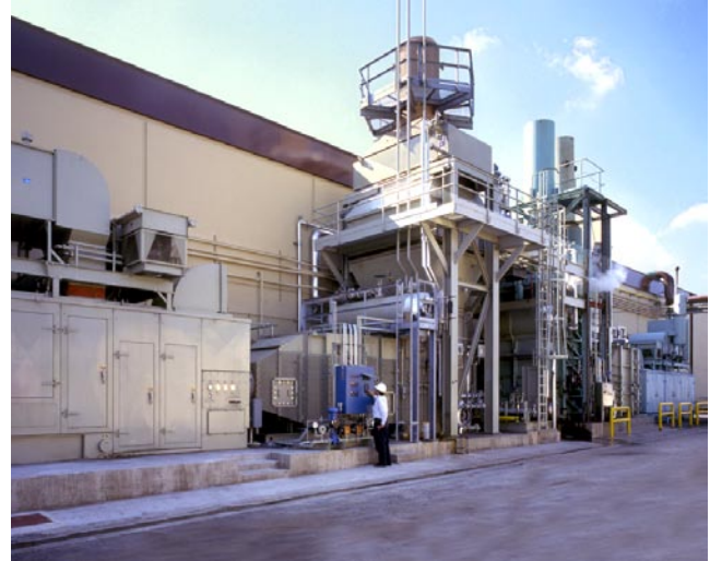
Taurus 60 Gas Turbine Generator Set
