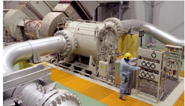
Titan Compressor Set with C65 Compressor
